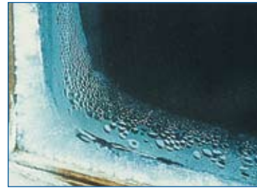
Window condensation can fuel mold growth.
